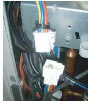
Compressor Wire Connection
