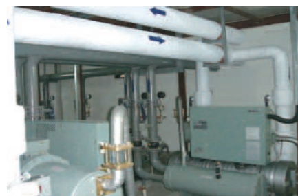
Machine Room for Conventional Central Water-source Unit
